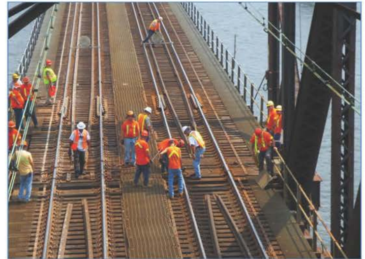
Amtrak crew manually opening the movable bridge span to accommodate marine traffic.
