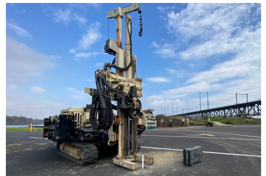
The Amtrak Environmental team uses a geoprobe to take soil samples from specific locations at defined depths. Geoprobos collect a continuous soil sample which is then analyzed for various environmental contaminants. Once the sample is taken, the borings are filled with backfill to restore the ground surface back to its pre-condition.
