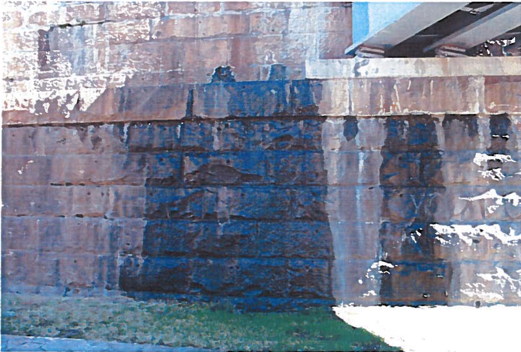
Extensive leakage & leaching at Adams Street
