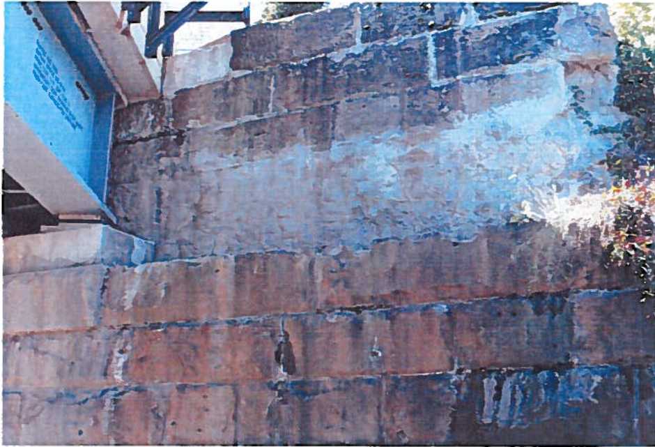
Unightly, modifications & deterioration at Adams Street
