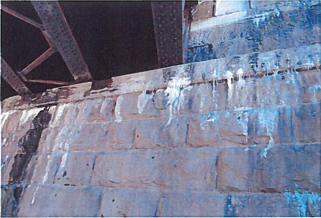
Leaching, concrete cap, & modified plate girder at Stokes.
