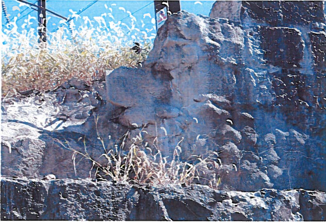
Severe abutment stone deterioration at Adams Street
