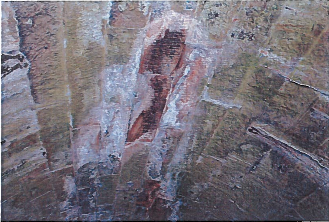
Leaching, deterioration & discoloration along ceiling of Freedom overpass
