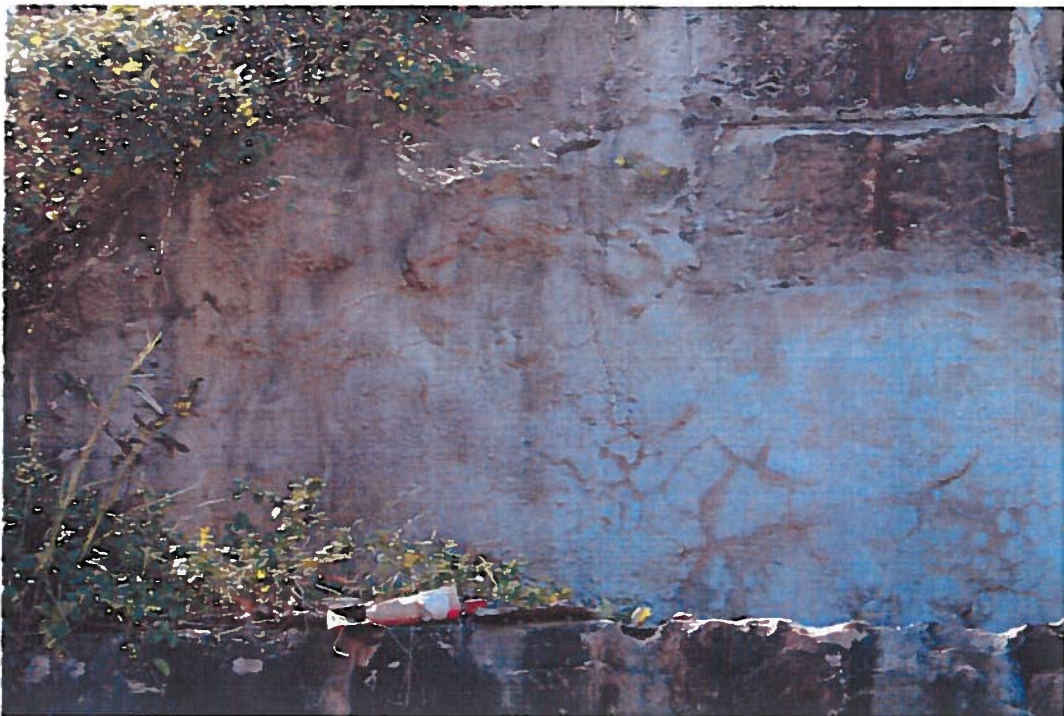
Deteriorated patching of chop-outs at Adams Street
