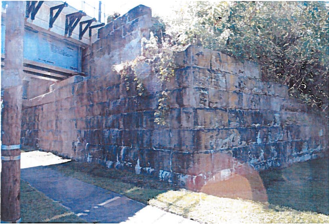
Chop-down modifications, leaching & deterioration at Adams Street
