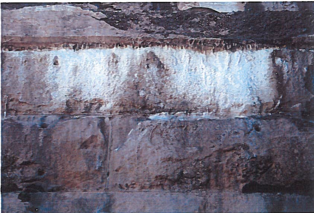
Leaching & deterioration at Stokes abutment
