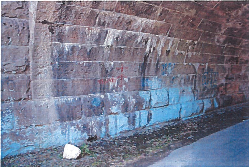
Leaching & discoloration within Centennial overpass
