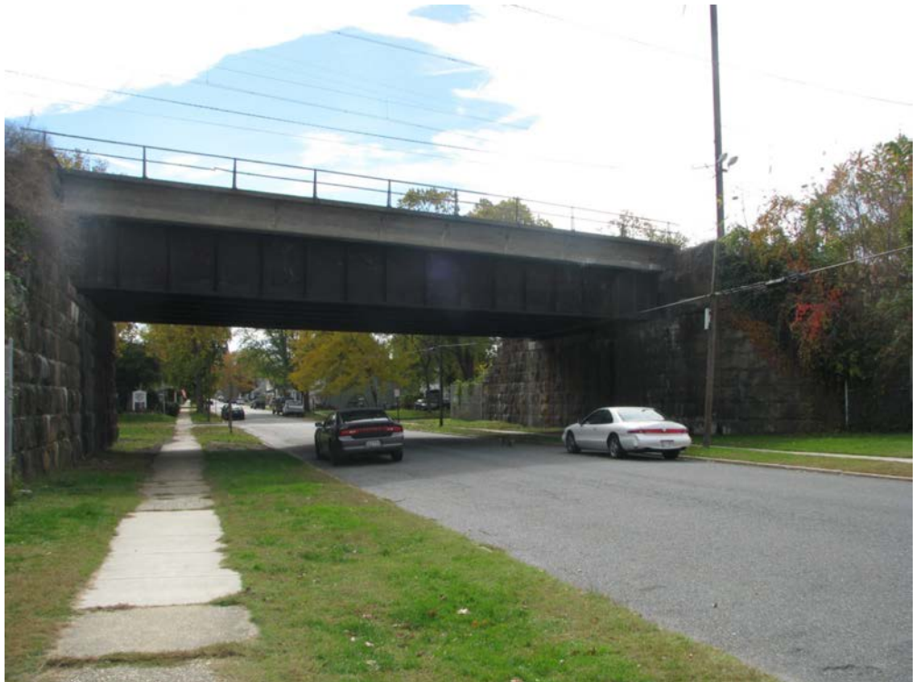
North Stokes Street Undergrade Bridge (MP 60.56): view of the railroad west side, 12 which will be altered via removing a portion of the existing stone masonry abutment and building a new concrete abutment; looking south.
