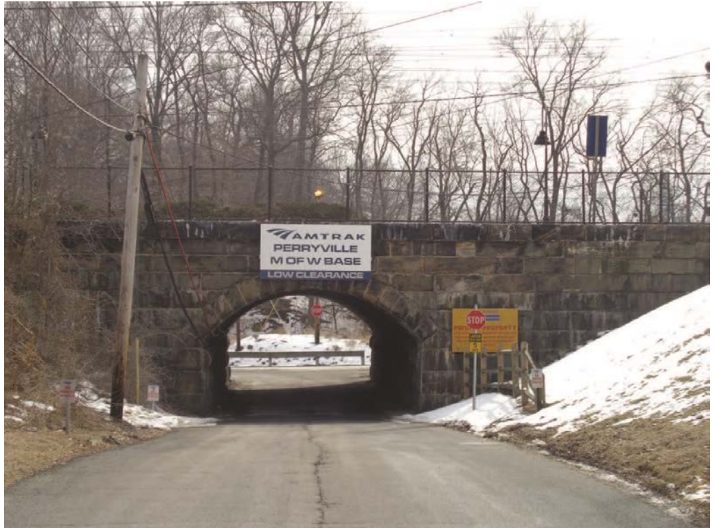
Perryville Railroad Station Undergrade Bridge (MP 59.39): View of the ashlar stone tunnel located east of the Perryville Railroad Station; looking south.
