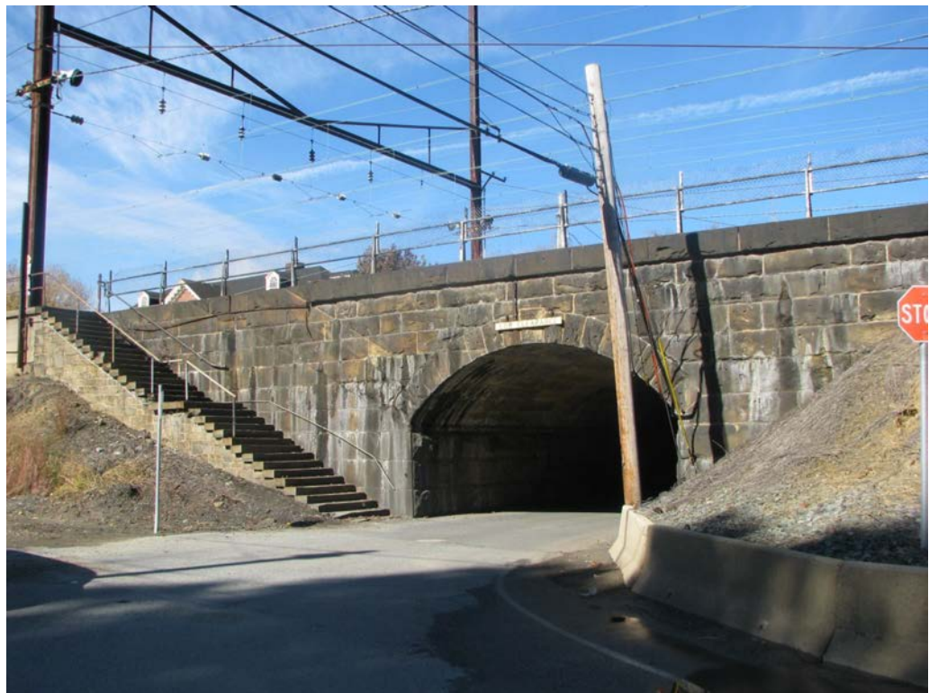
Perryville Railroad Station Undergrade Bridge (MP 59.39): view of the east side, which will be extended with a precast concrete culvert. 26
