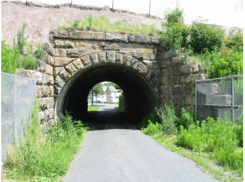
North Freedom Lane Undergrade Bridge (MP 60.51): view of the railroad east side, 11 which will be altered via removing the existing stone-arch culvert and replacing it with a precast concrete culvert; looking north.
