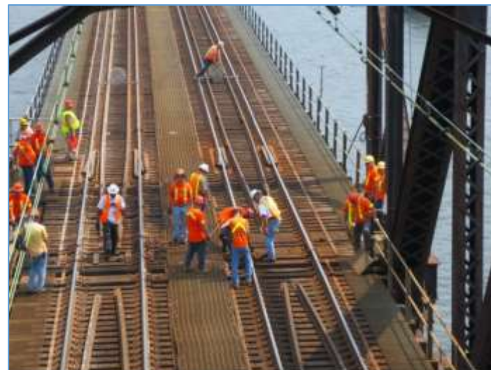
Amtrak crew manually opening the movable bridge span to accommodate marine traffic.
