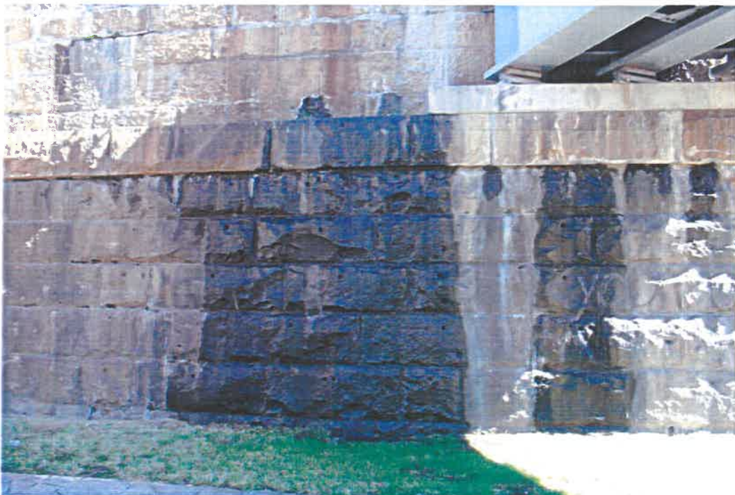
Extensive leakage & leaching at Adams Street
