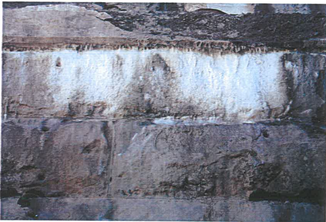
Leaching & deterioration at Stokes abutment
