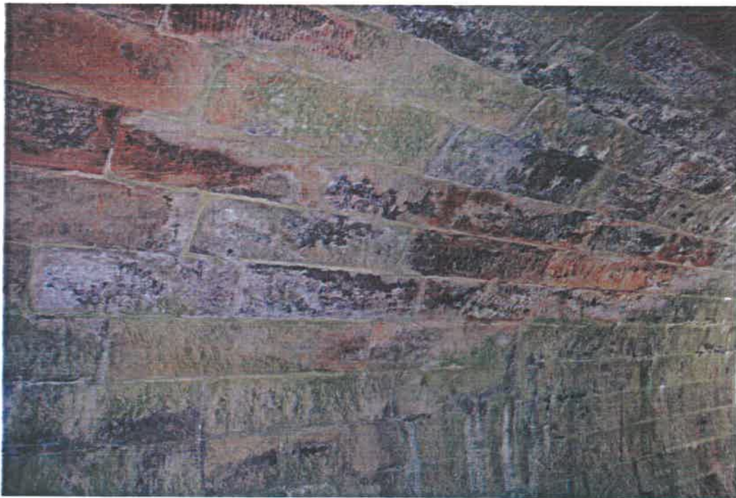
Leaching & discoloration within Freedom overpass
