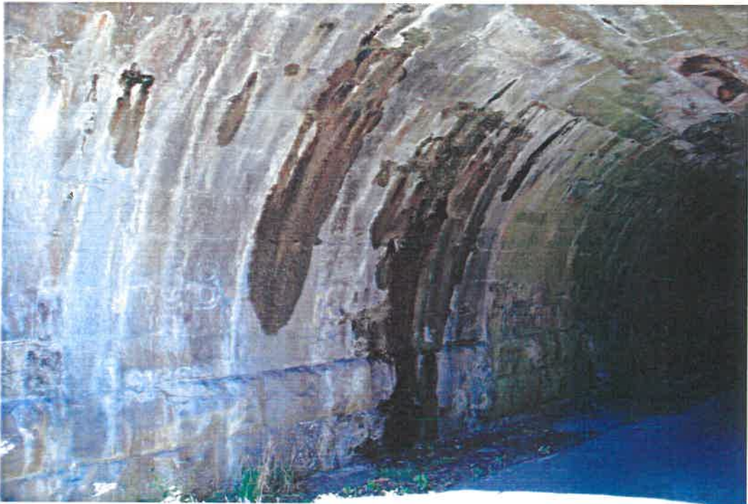
Leaching & leaking within Freedom overpass
