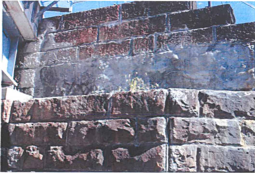
Unsightly modification patching & severe leaching at Adams Street
