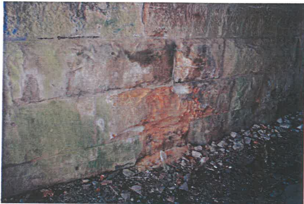
Leaching, discoloration & deterioration within Centennial overpass
