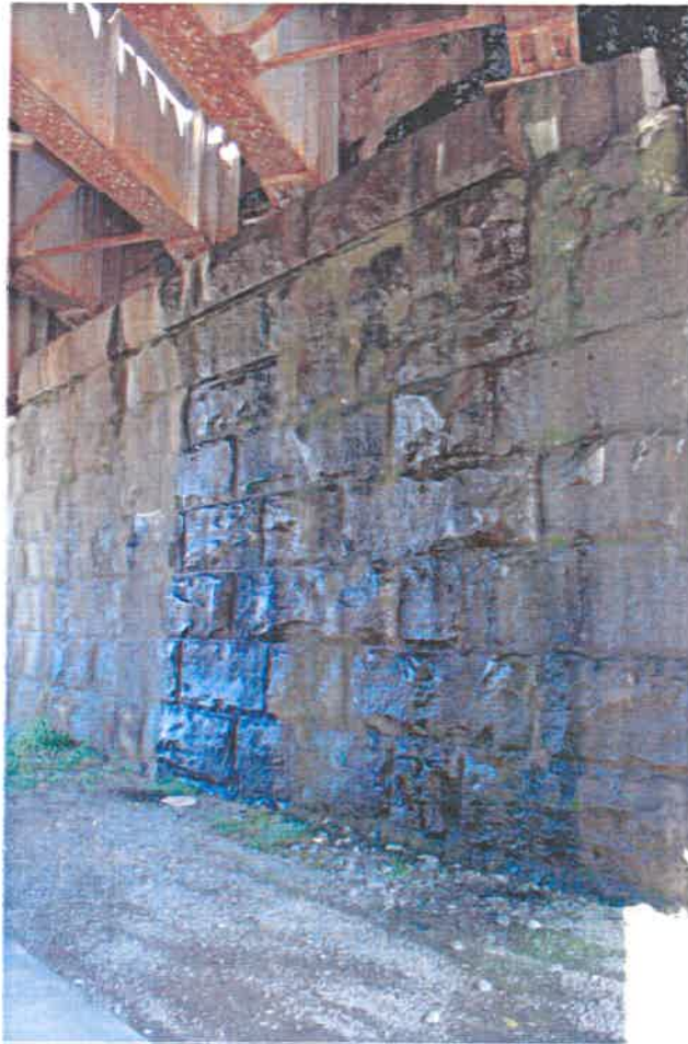
Abutment leakage, deterioration & discoloration at Juniata Street
