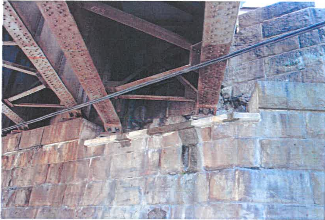
Abutment chop-down, chop-out, capping & leakage at Juniata Street
