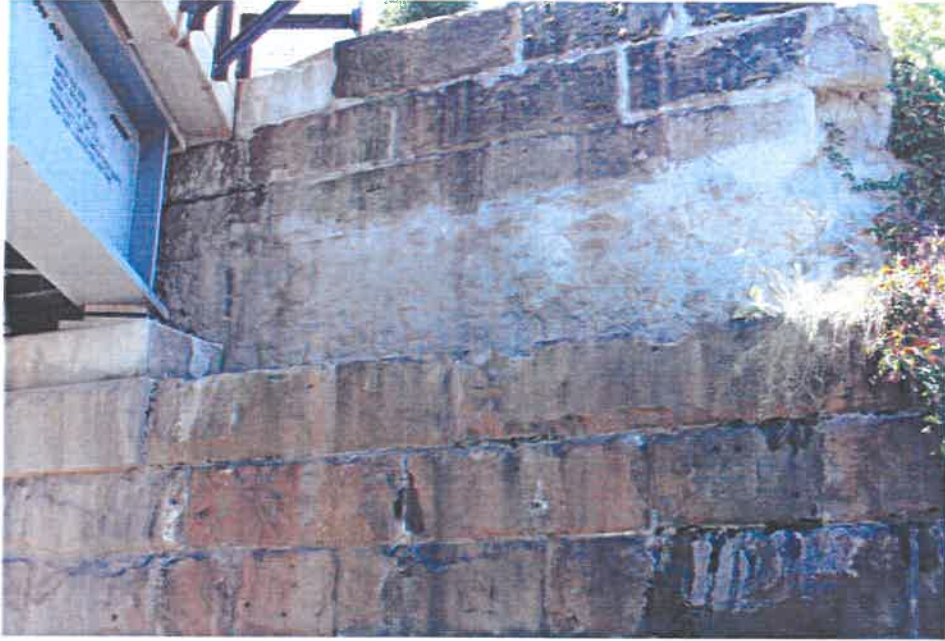
Unsightly, modifications & deterioration at Adams Street
