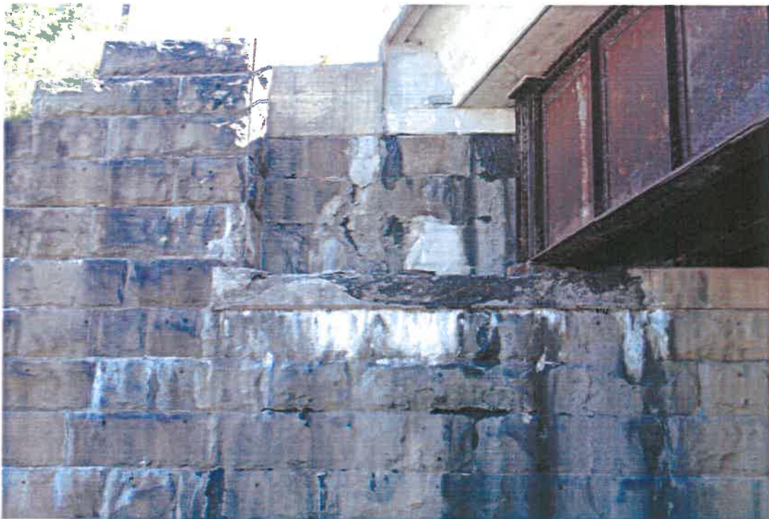
Chop-down, chop-out, concrete caps, plate girder modification, leaching & discoloration at Stokes abutment
