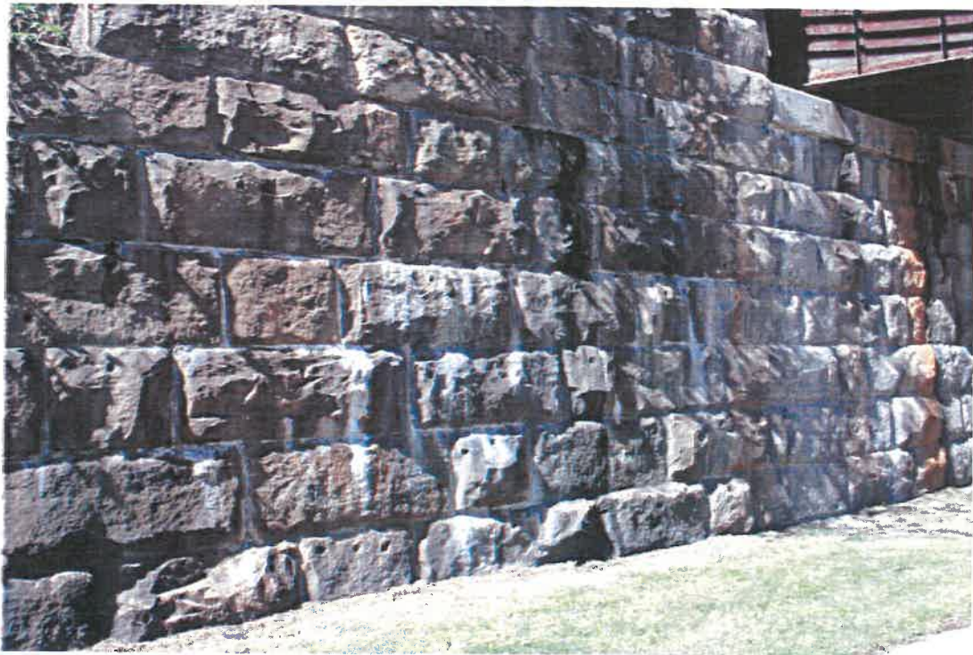
Leaching & leaking at Stokes Street abutment
