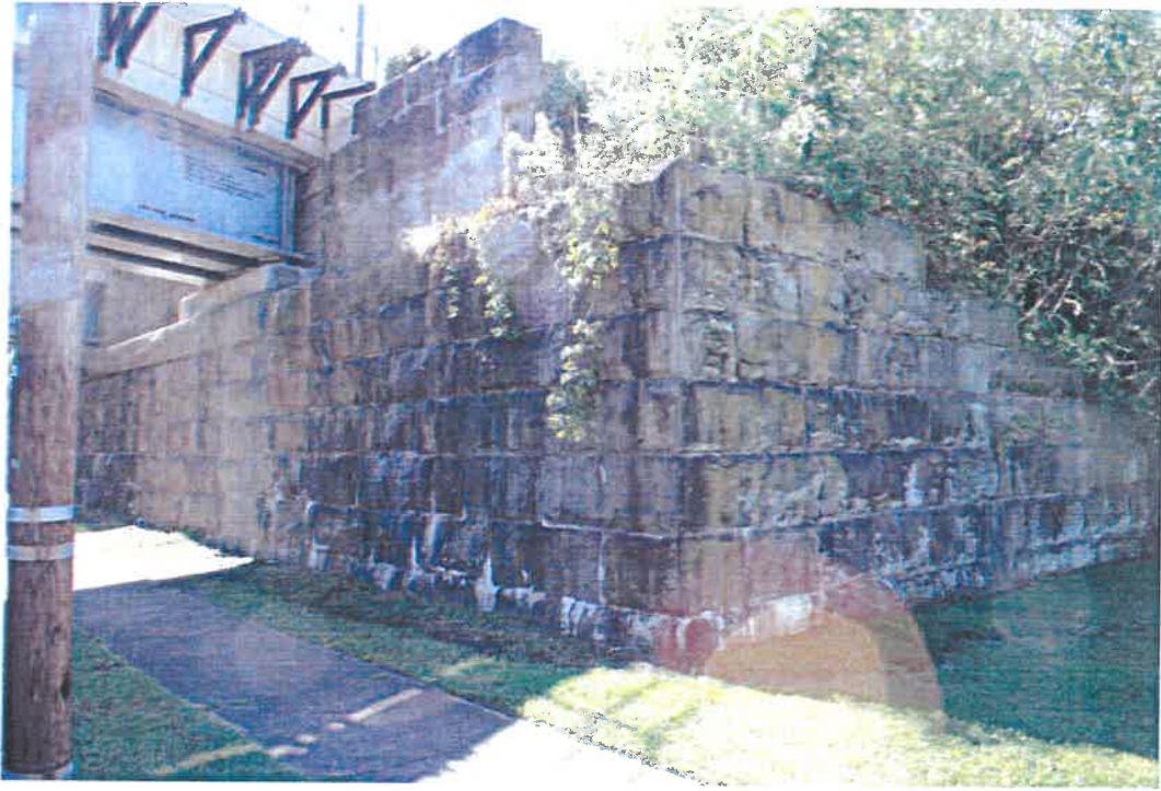
Chop-down modifications, leaching & deterioration at Adams Street
