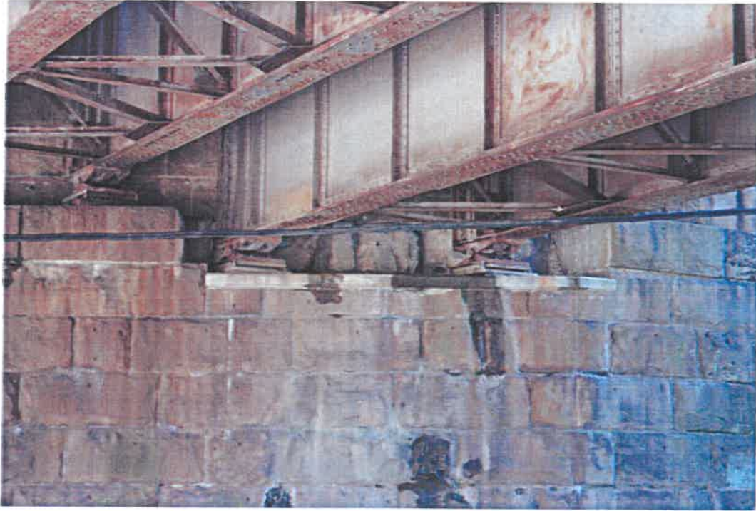
Abutment chop-down, capping & leakage at Juniata Street
