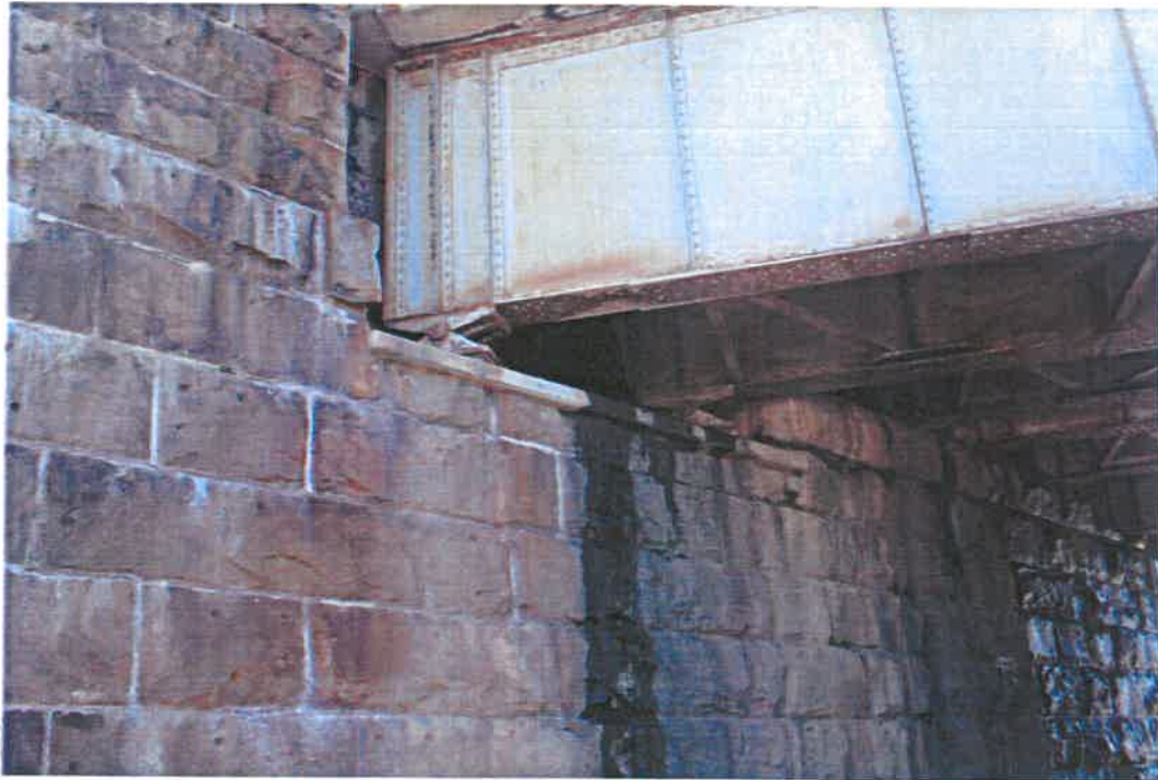
Abutment chop-down, capping & leakage at Juniata Street
