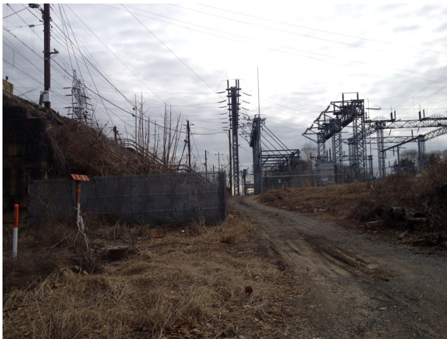
Electric substation located adjacent to south of railroad corridor in Perryville, view to the east.
