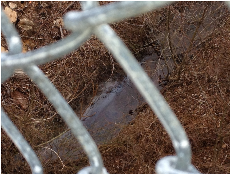
Petroleum-like sheen observed on standing water in ditch adjacent to the railroad, view to the east from the Firestone Road bridge.
