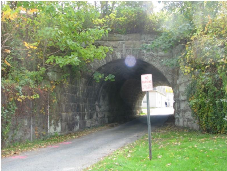
Photo 56: View looking south at the railroad west side of North Freedom Lane Undergrade Bridge (MP 60.51), which will be altered via construction of a precast concrete culvert.
