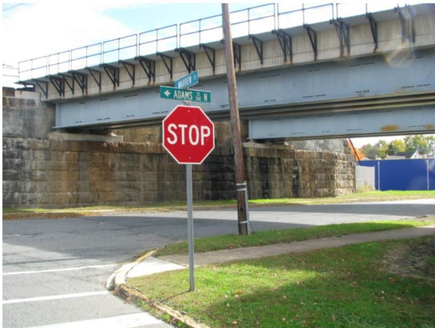
Photo 62: View looking southeast at the railroad west side of North Adams Street Undergrade Bridge (MP 60.69) that will be extended with a concrete abutment.
