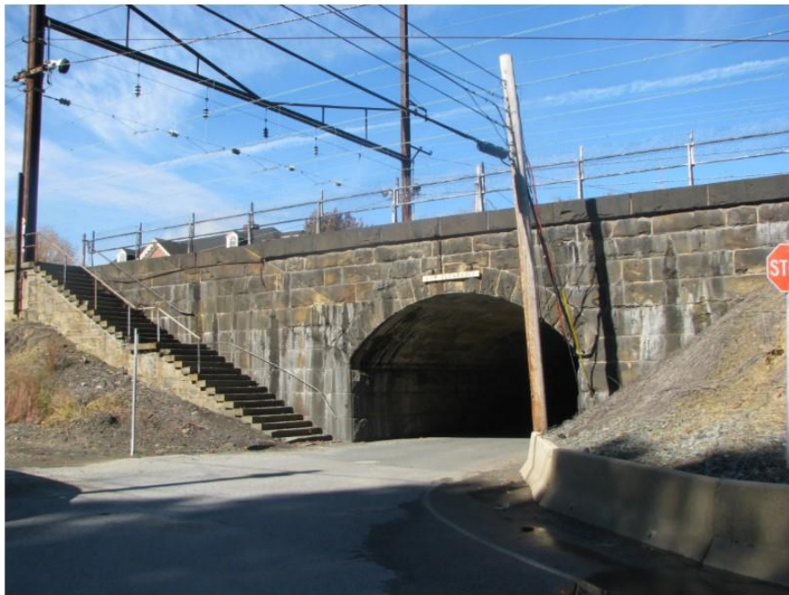
Photo 52: View looking at the east side of Perryville Railroad Station Undergrade Bridge (MP 59.39) that will be extended with a precast concrete culvert.
