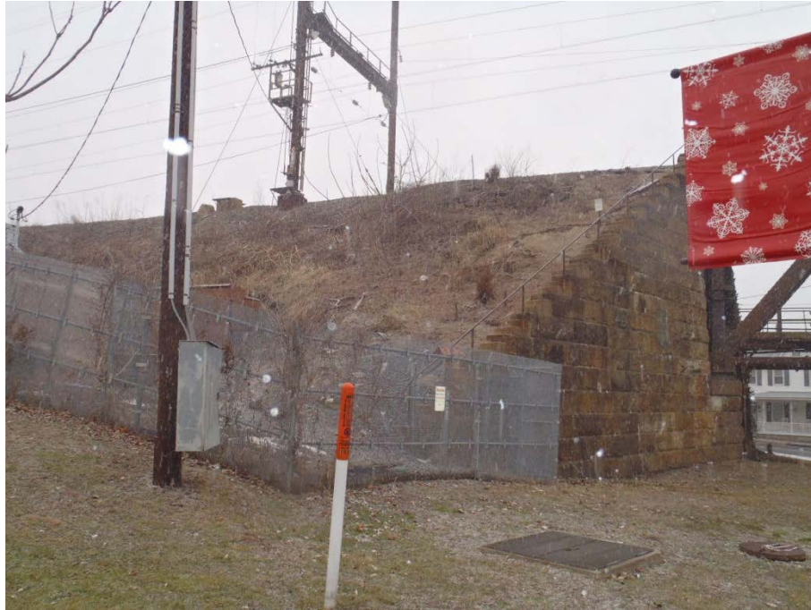
Photograph 3: General view of embankment supporting railroad and railroad bridge over St. John Street, facing southwest; Note the presence of multiple underground utilities within the vicinity of the berm.
