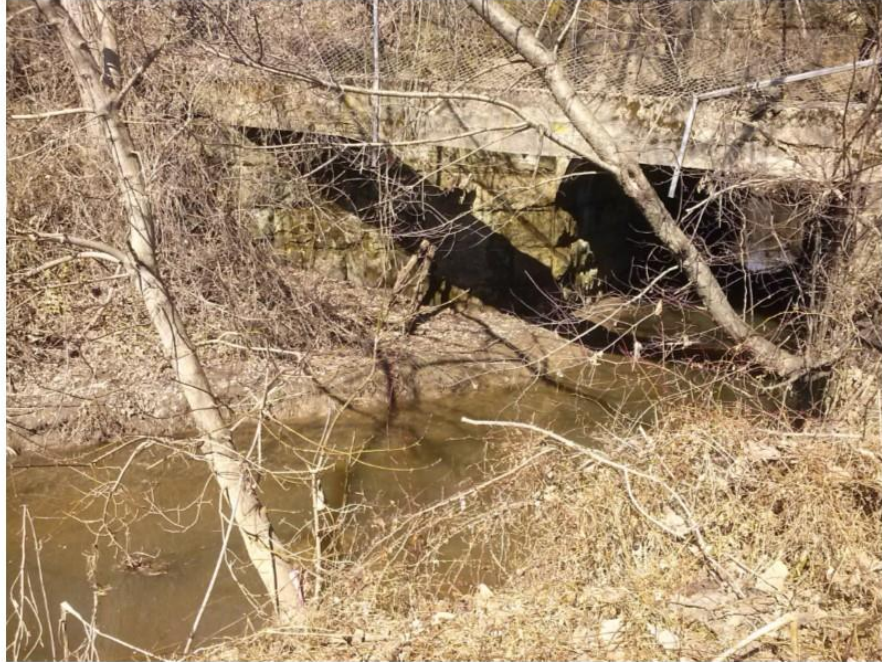
Photo 64: View looking northeast at the railroad east side Lily Run Undergrade Bridge (MP 60.85) which will be spanned over by a multi-girder bridge.
