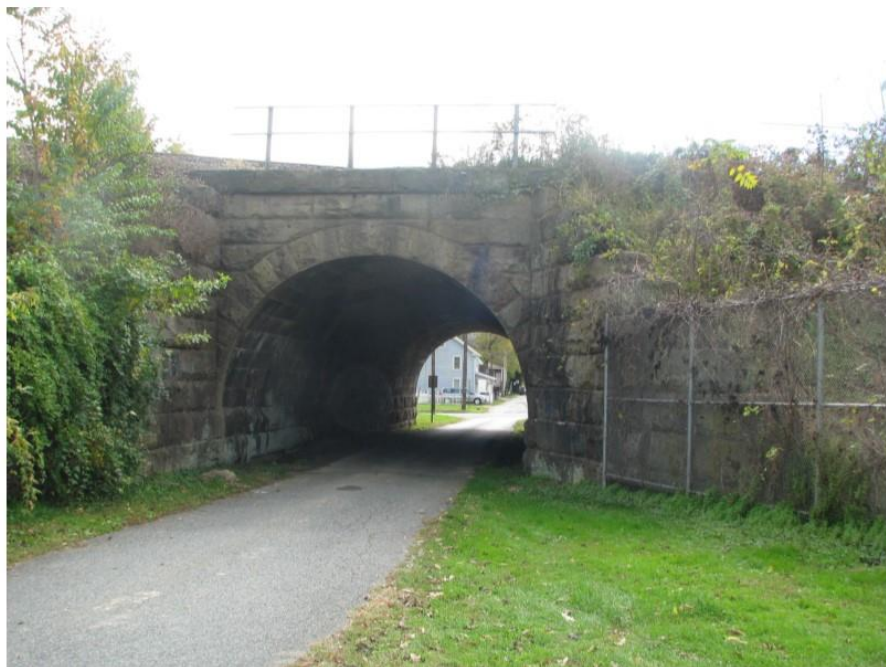
Photo 60: View looking south at the railroad west side of Centennial Lane Undergrade Bridge (MP 60.61), which will be extended with a precast concrete culvert.
