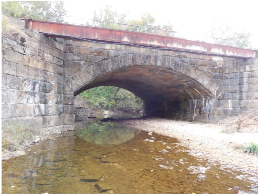
Photo 51: View looking northwest at the east side of the Mill Creek Undergrade Bridge (MP 59.00) that will be extended with a precast concrete culvert.
