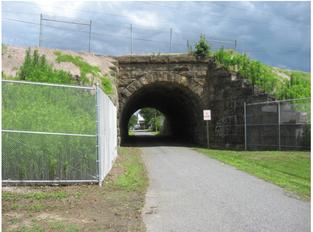
View looking north at the Centennial Lane Undergrade Bridge (MP 60.61), one of nine undergrade bridges considered historically significant in relation to the Susquehanna River Rail Bridge. 3
