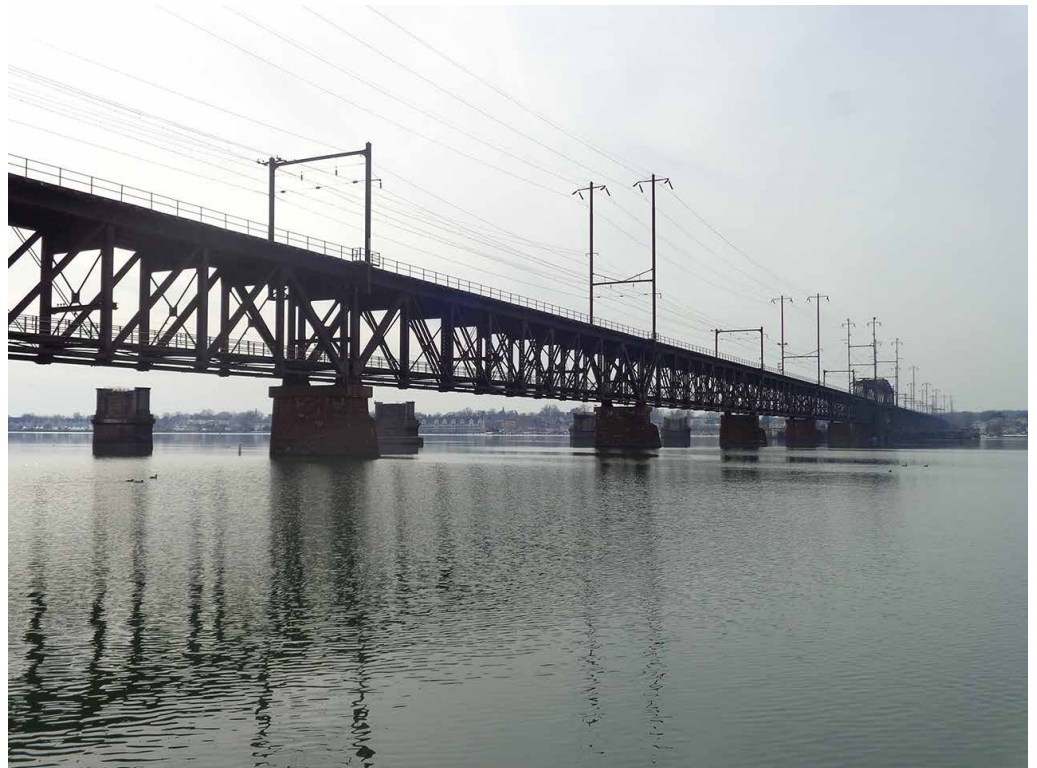
View looking west at the Susquehanna River Rail Bridge from the Perryville waterfront. 2
