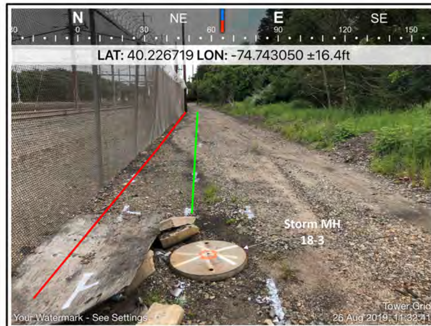
Photo 2: The photo shows storm manhole 18-3, the approximate location of the 5.5-foot diameter storm line next to the fence and an electric line. The approximate photo location, direction the photo was taken, and the date and time of the photo is presented.
