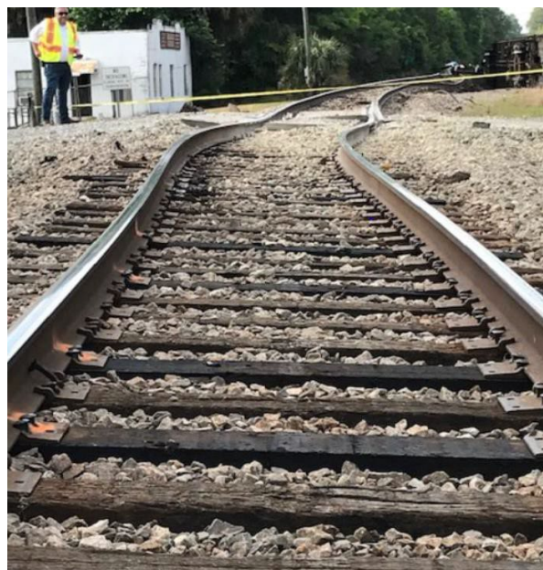
Figure 22 Track Misalignment in a Curve with Road Crossing
