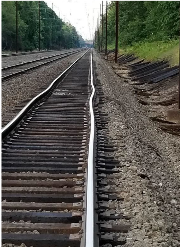
Figure 23 Track Misalignment After Out-of-Face Tie Renewal
