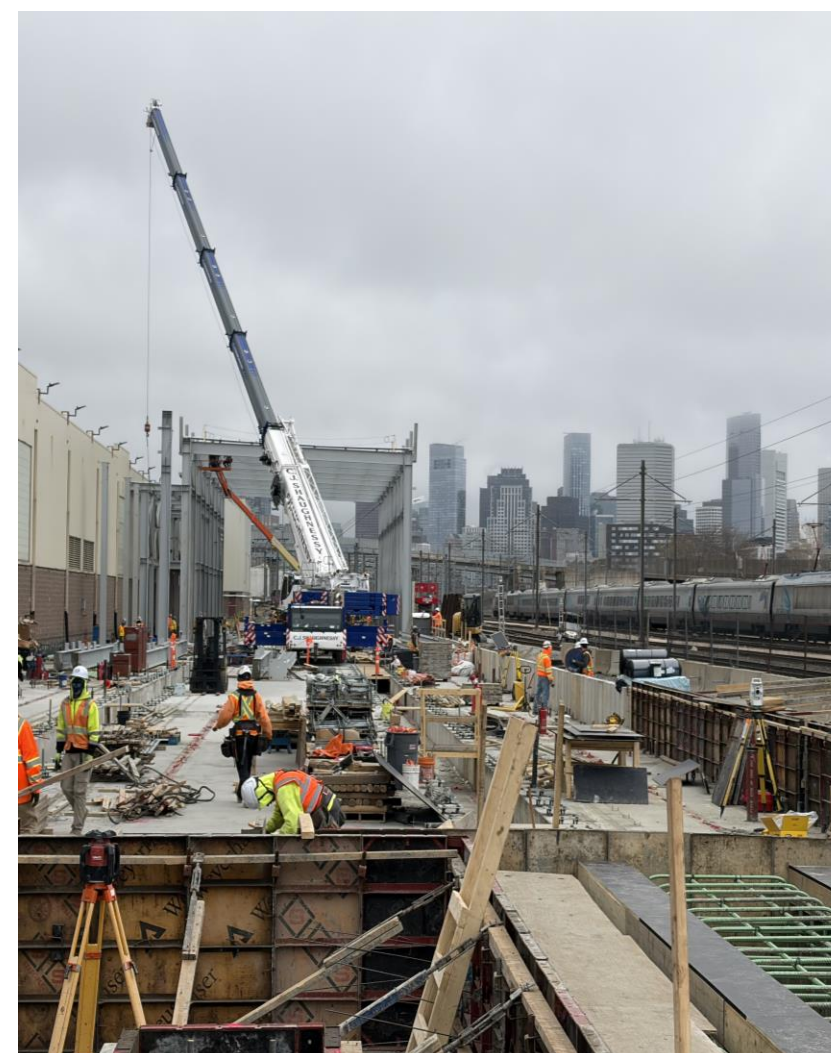
Southampton Yard, Boston, MA Made significant progress on concrete pours and began erection of steel for M&I facility
