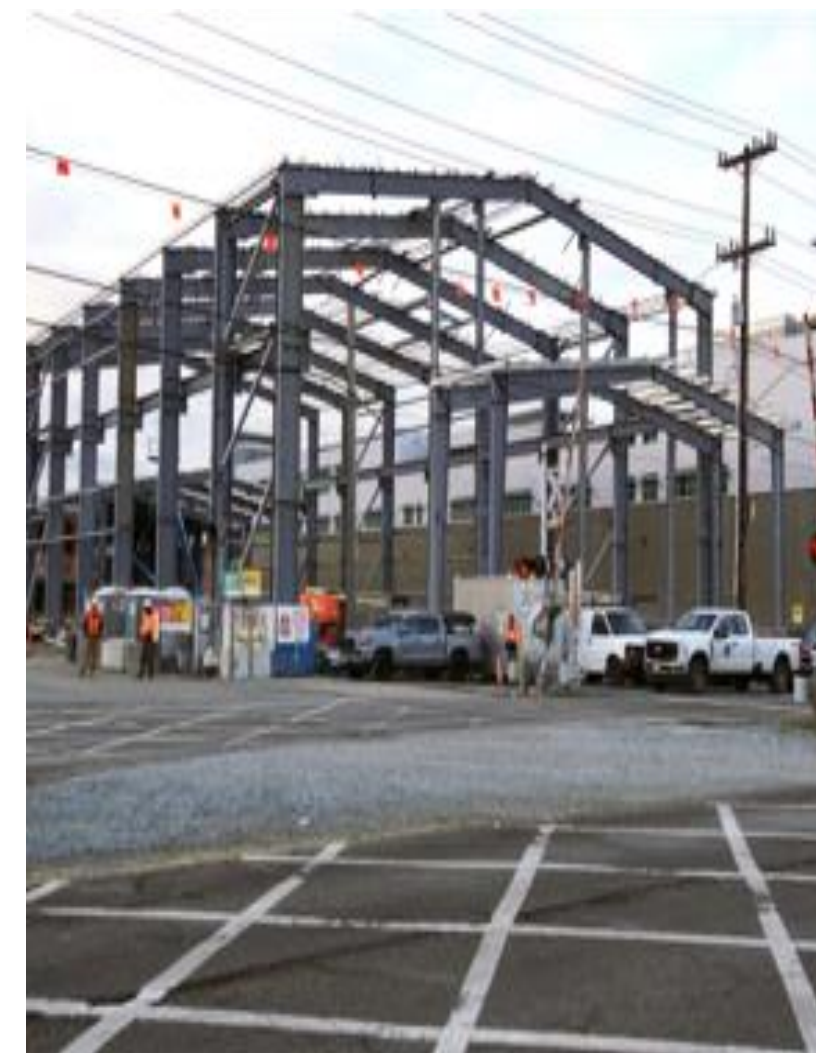
Seattle Yard Seattle, WA Topped out steel structure for new M&I facility
