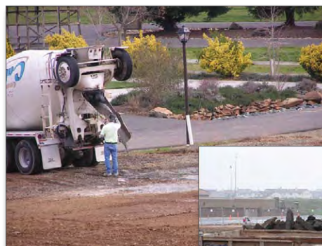
Figure 1. Chute washwater being dumped on the ground
