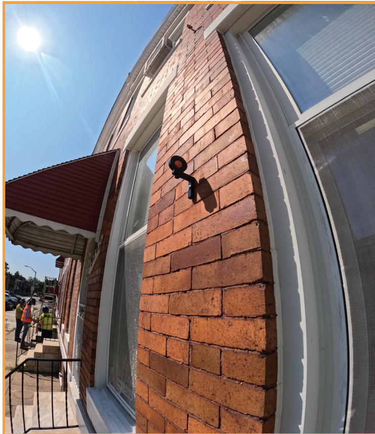
Installed tilt monitor
