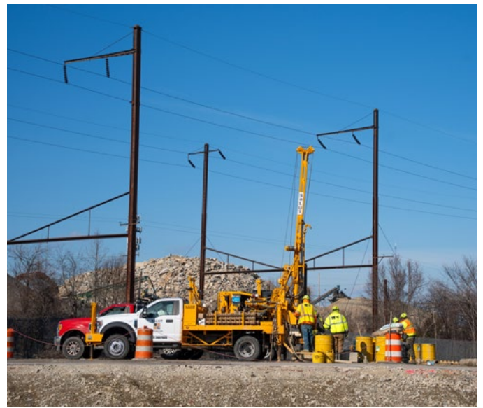
Soil boring investigations at the future South Portal site or southern entrance of the tunnel (near North Payson Street)
