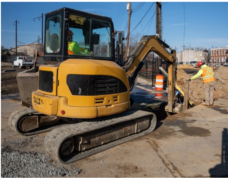
Crews use an excavator to prepare the ground for the installation of temporary waterlines
