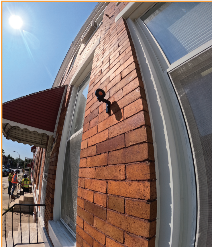
Installed tilt monitor
